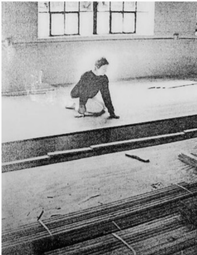
September 20, 1990 Mary-Liz Humphrey checks the rooms new sprung flooring. The revamping of the old building was a joint effort of the rec commission and the town of Elkton.
